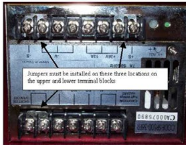
Figure 2 - Power Supply Unit Terminal Jumpers
