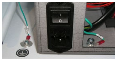
Figure 1 - Power Supply Ground Wires
