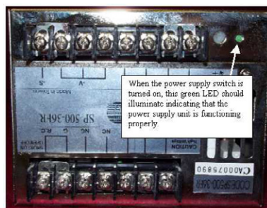
Figure 3 - Power Supply Indicator LED
