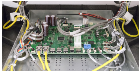
Figure 1 - Main PCB Installed
