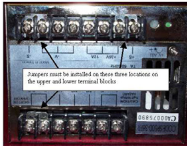
Figure 2 - Power Supply Unit Terminal Jumpers
