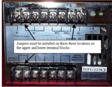
Figure 2 - Power Supply Unit Terminal Jumpers
