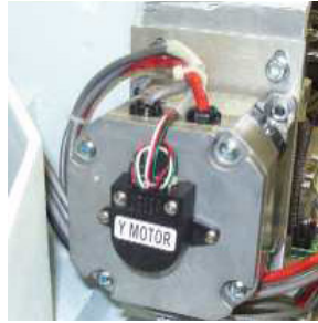
Figure 3 - Harnessing Routed Under Y-Motor
