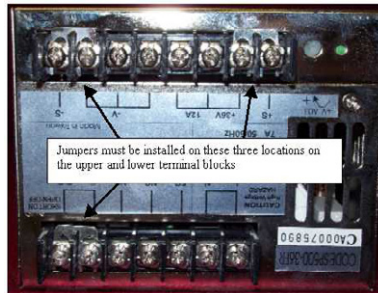
Figure 2 - Power Supply Unit Terminal Jumpers
