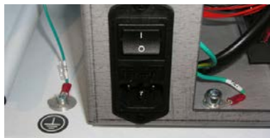
Figure 1 - Power Supply Ground Wires
